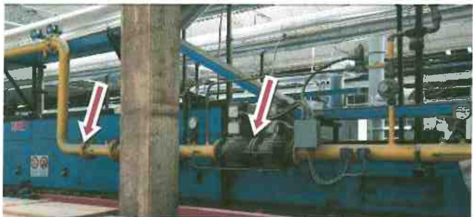
Rampa gas Forno 2
