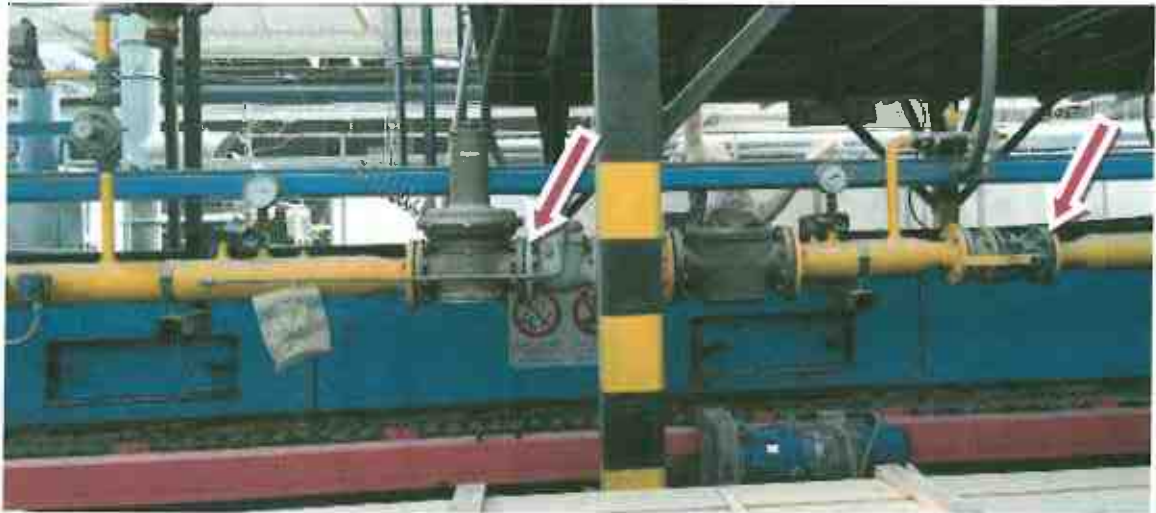
Rampa gas Forno 2
