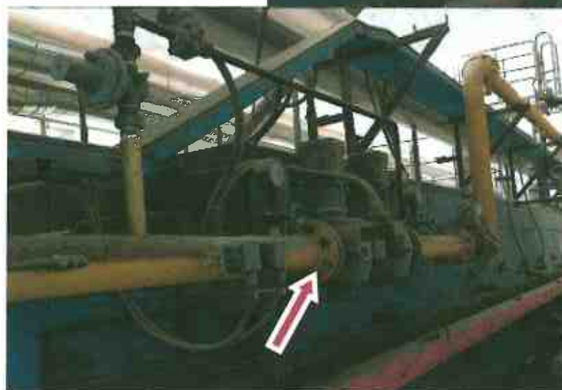
Rampa gas Forno 1
