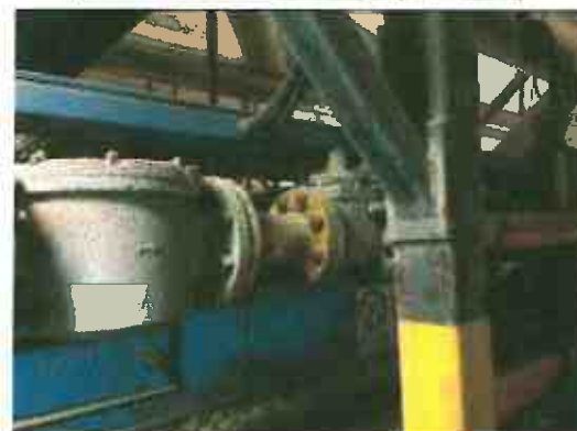
Rampa gas Forno 1
