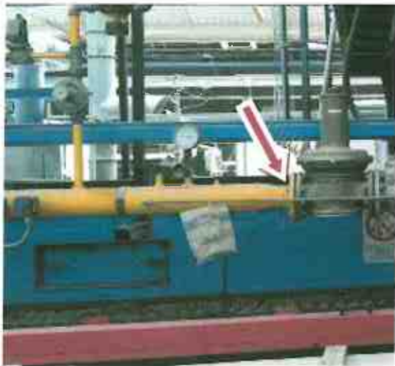
Rampa gas Forno 2
